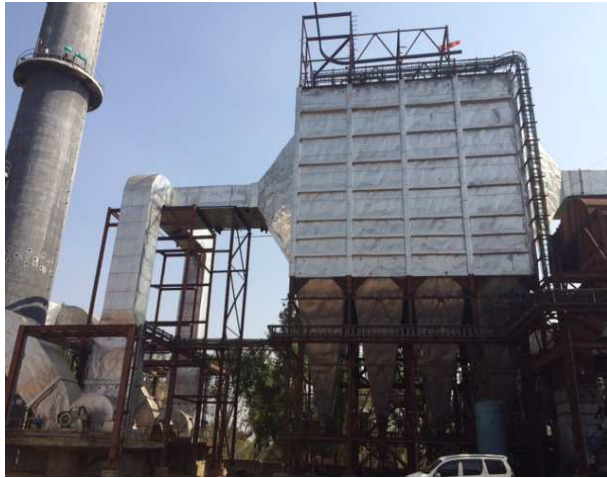
ESP for New Boiler
