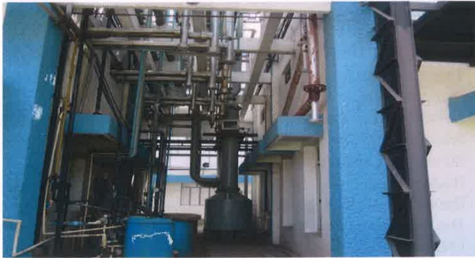
View of plant Area and Scrubber
